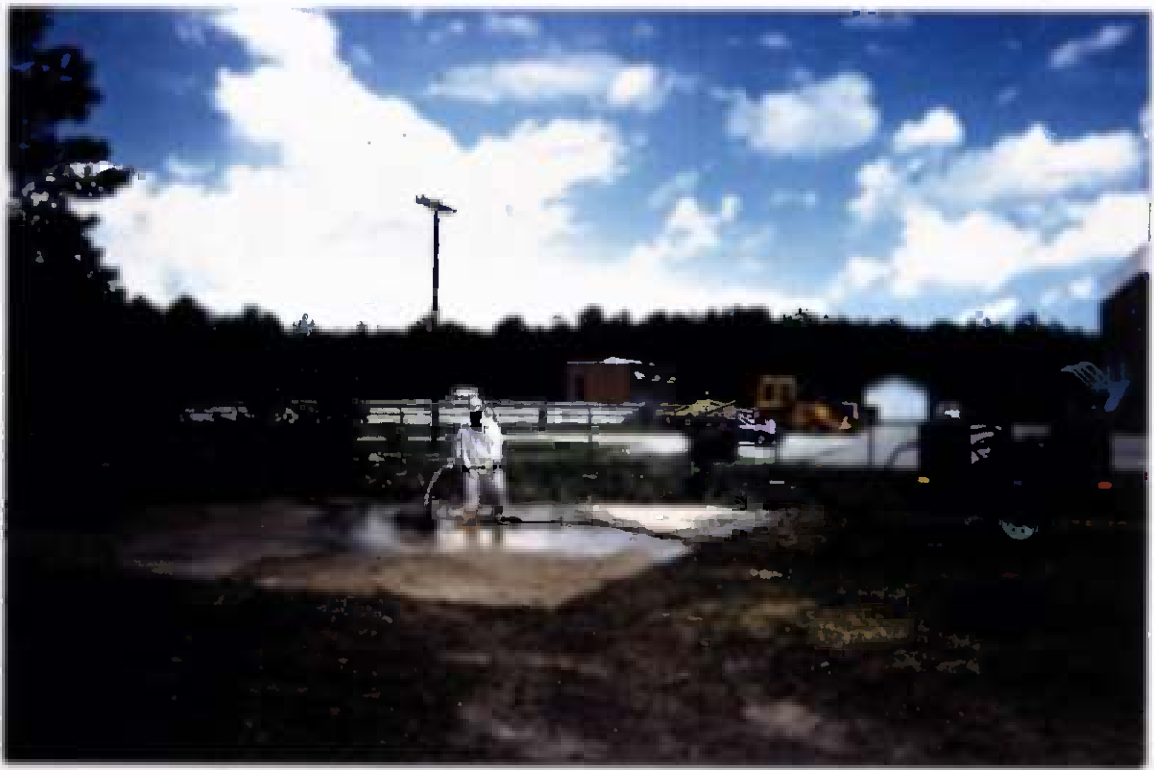
Project No. 16207 Contract No. N62470-93-D-3032 Delivery Order: 0023 Location : Area 2 Description: scabbling / scarify north mixing pad
