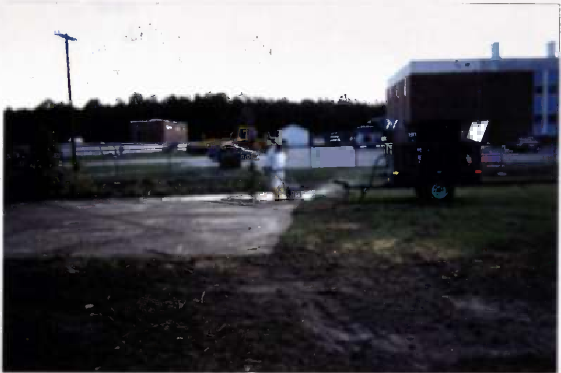
Project No. 16207 Contract No. N62470-93-D-3032 Delivery Order: 0023 Location : Area 2 Description: scabbling / scarify north mixing pad
