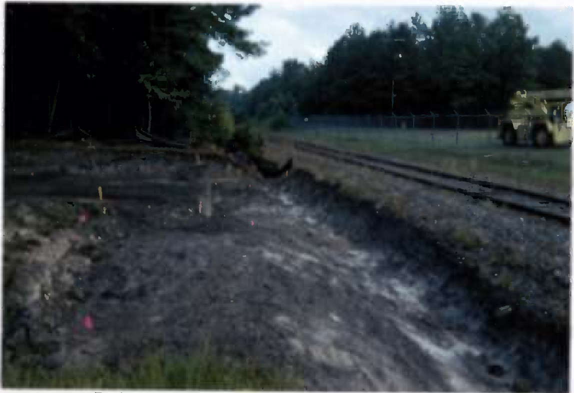
Project No. 16207 Contract No. N62470-93-D-3032 Delivery Order: 0023 Location : Area 2 Description: completion of northern excav., flagging represents confirmation sample locations
