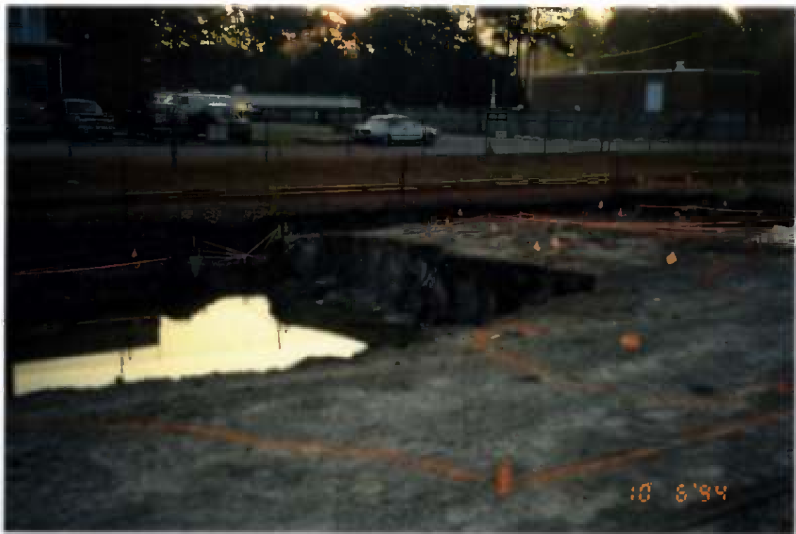
Project No. 16207 Contract No. N62470-93-D-3032 Delivery Order: 0023 Location : Area 1 Description: excav. area 1 after sample delineation, stakes & paint flagging
