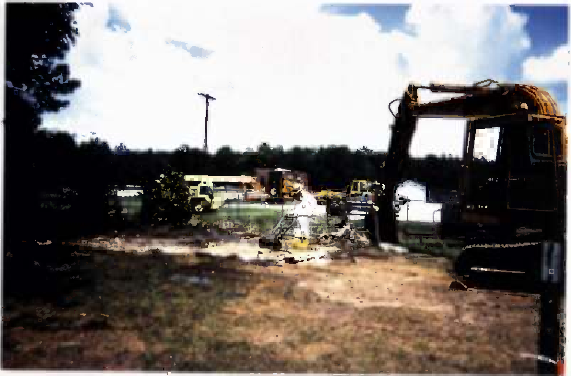
Project No. 16207 Contract No. N62470-93-D-3032 Delivery Order: 0023 Location : Area 2 Description: scabbling / scarify north mixing pad, scabbling underside of concrete
