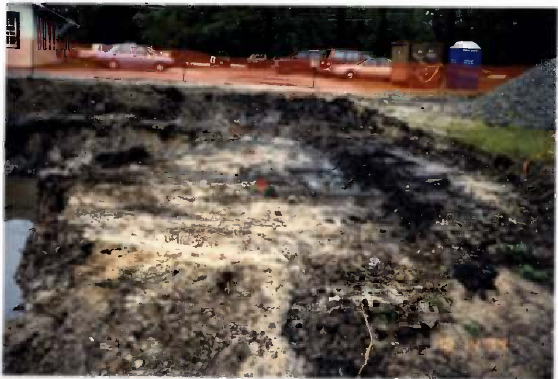
Project No. 16207 Contract No. N62470-93-D-3032 Delivery Order: 0023 Location : Area 1 Description: excav. area 1 after phase 2, flagging represents confirmation sample location
