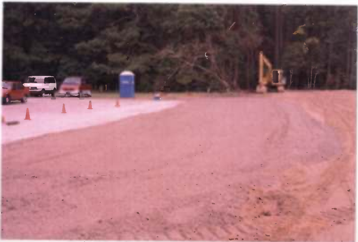
Project No. 16207 Contract No. N62470-93-D-3032 Delivery Order: 0023 Location : Area 3 Description: backfilling operations, stone used for areas under water
