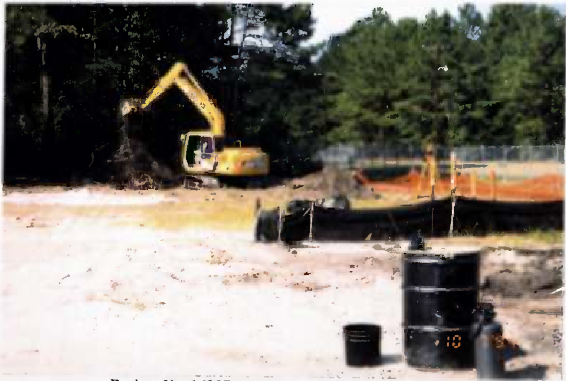
Project No. 16207 Contract No. N62470-93-D-3032 Delivery Order: 0023 Location : Area 2 Description: initial excav. of northern area, survey instrmnt. for level control
