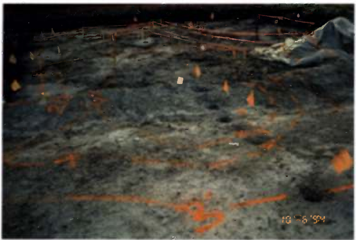
Project No. 16207 Contract No. N62470-93-D-3032 Delivery Order: 0023 Location : Area 1 Description: excav. area 1 after sample delineation, stakes & paint flagging
