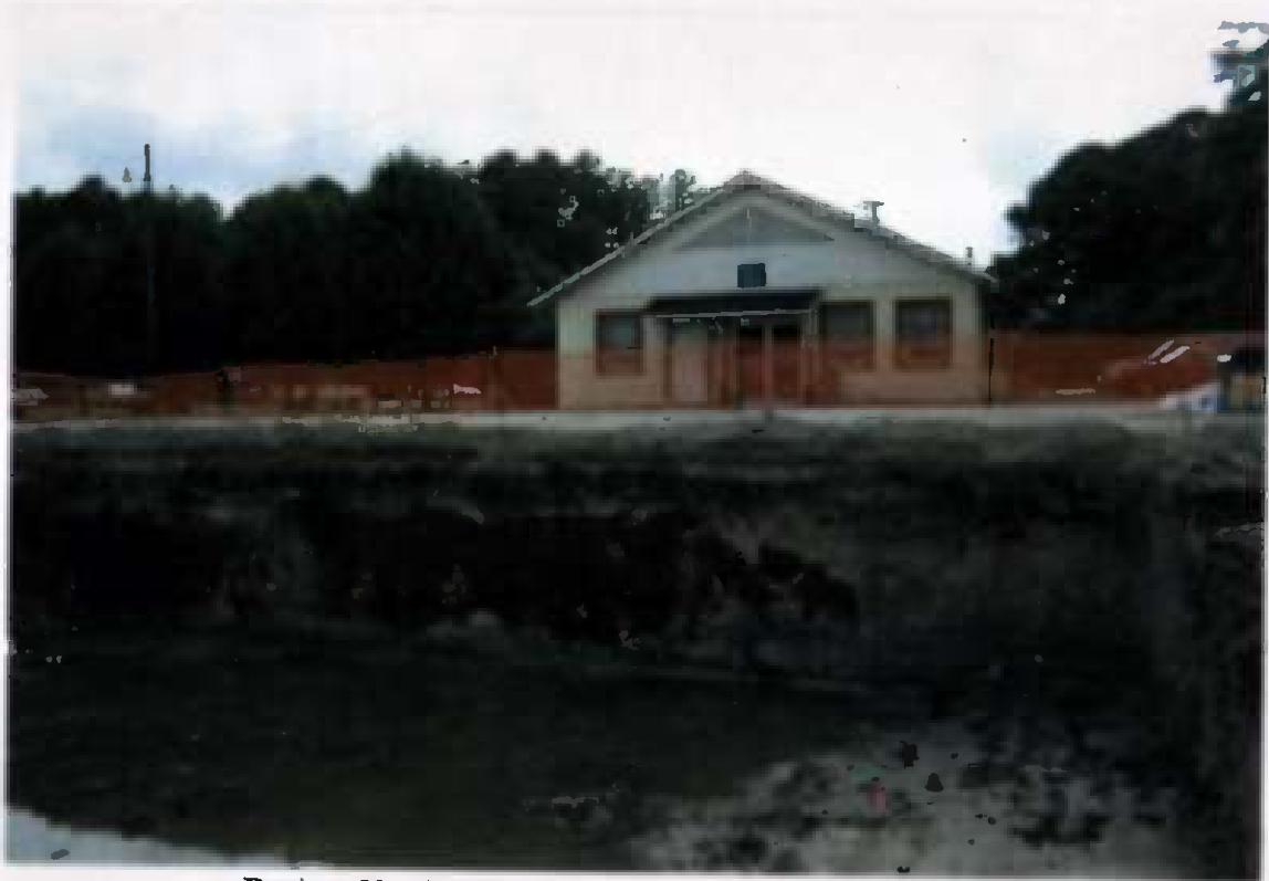
Project No. 16207 Contract No. N62470-93-D-3032 Delivery Order: 0023 Location : Area 1 Description: excavation of area 1 with petroleum contamination
