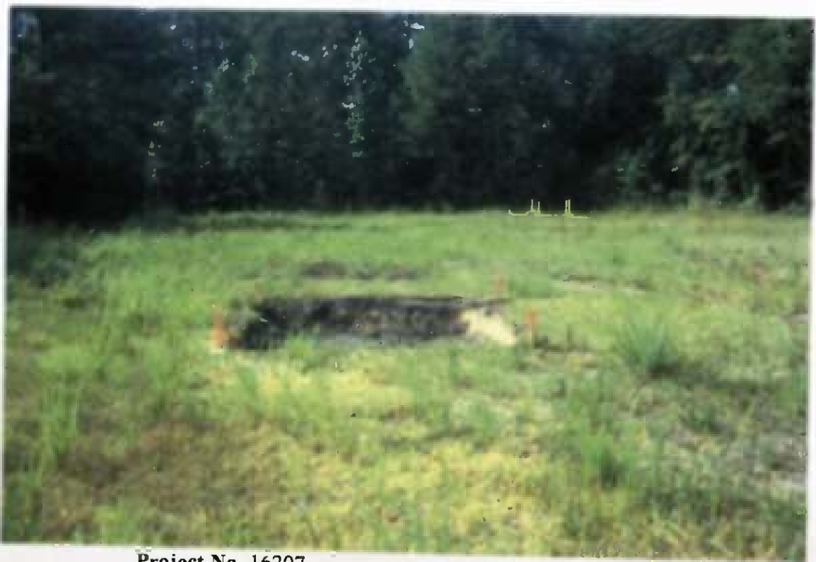
Project No. 16207 Contract No. N62470-93-D-3032 Delivery Order: 0023 Location : Area 3 Description: excav. area 3 on east side of tracks upon completion
