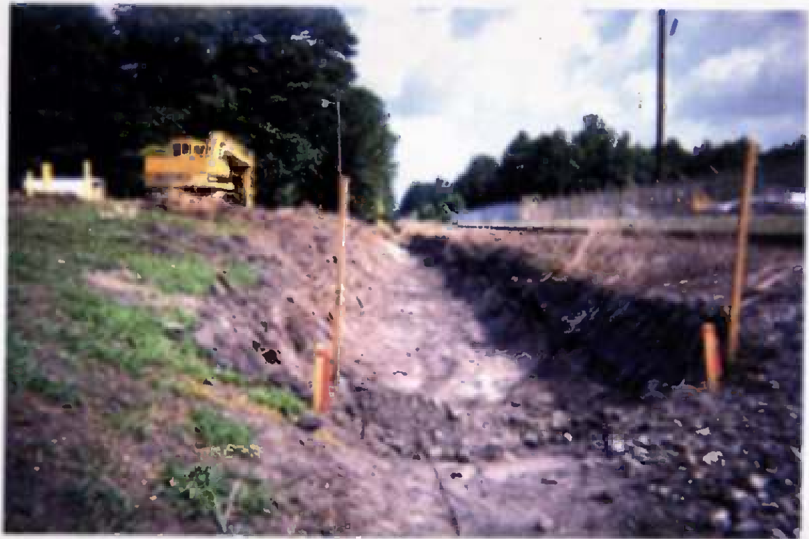
Project No. 16207 Contract No. N62470-93-D-3032 Delivery Order: 0023 Location : Area 2 Description: excav. of drainage ditch north of area 2
