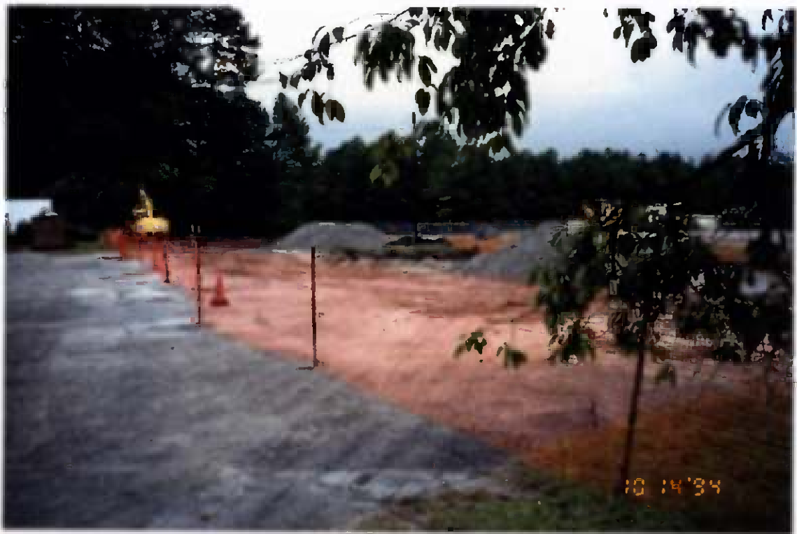
Project No. 16207 Contract No. N62470-93-D-3032 Delivery Order: 0023 Location : Area 3 Description: backfilling operations, stone used for areas under water
