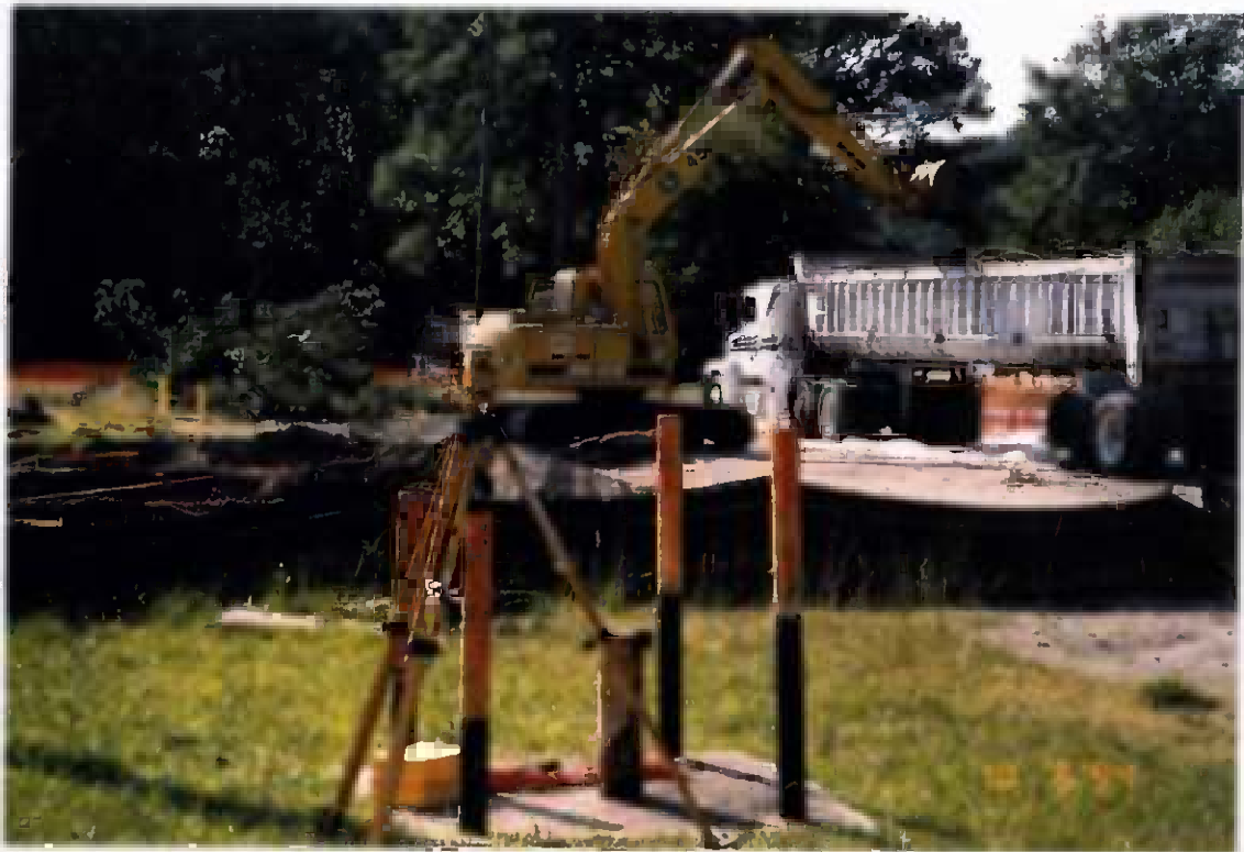
Project No. 16207 Contract No. N62470-93-D-3032 Delivery Order: 0023 Location : Area 1 Description: 2nd excavation of area 1 direct load, survey instrmnt. for level control
