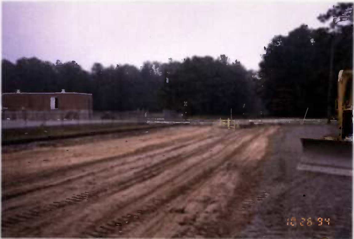
Project No. 16207 Contract No. N62470-93-D-3032 Delivery Order: 0023 Location : Area 3 Description: backfilling operations, stone used for areas under water
