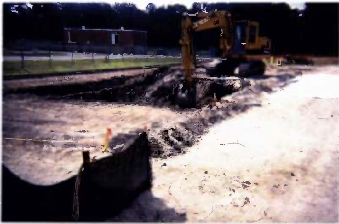
Project No. 16207 Contract No. N62470-93-D-3032 Delivery Order: 0023 Location : Area 1 Description: initial 6' excavation, soils were direct loaded into trucks , note drainage berm
