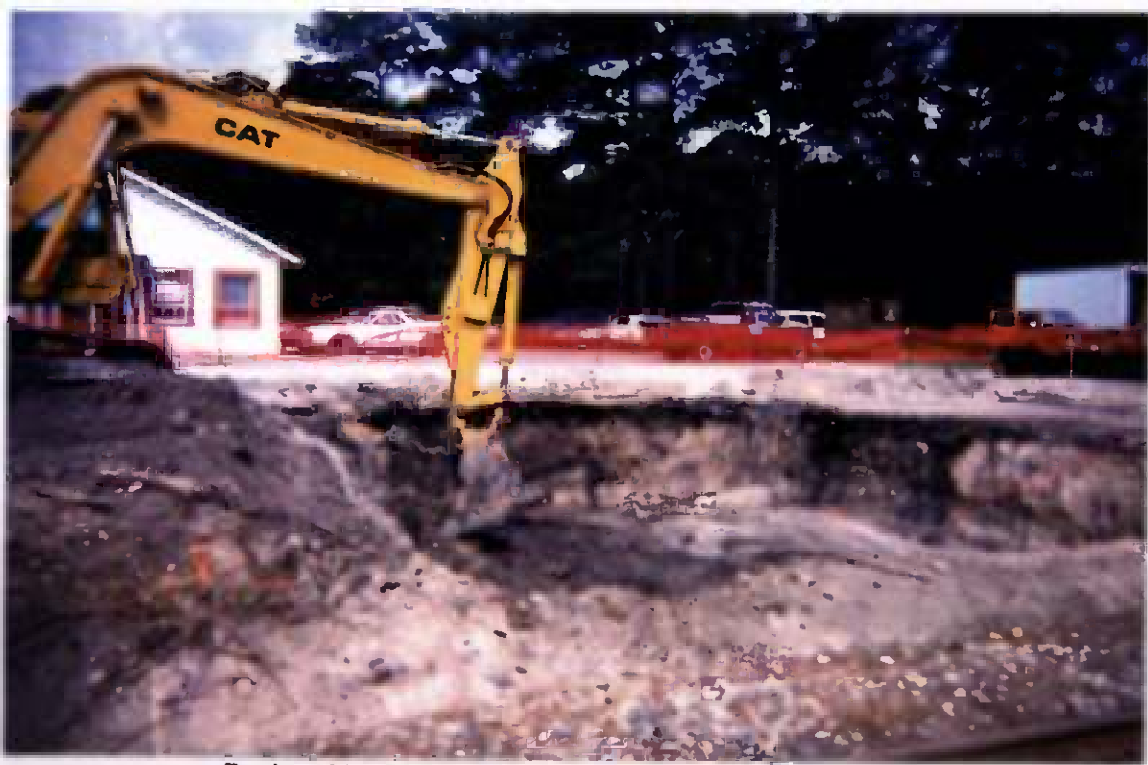
Project No. 16207 Contract No. N62470-93-D-3032 Delivery Order: 0023 Location : Area 1 Description: initial excavation of area 1, 6' excavation
