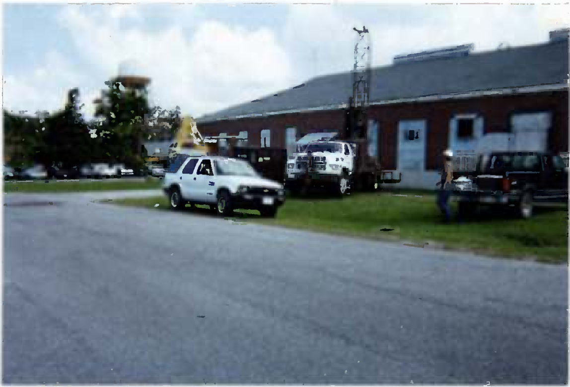
Photo # WP-3 Installing temporary intermediate well TW04IW on the south side of Building 25. The temporary wells were installed using hollow stem augers and a truck-mounted drill rig. This particular well was installed at a depth of 50 feet below ground surface.
