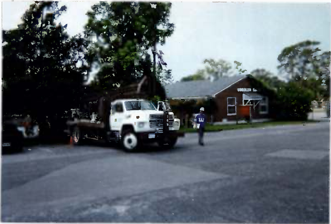
Photo # WP-4 Work proceeding at temporary well location TW15. This well was located west of Building 25. The cobbler shop (Building 43) can be seen in the photograph.
