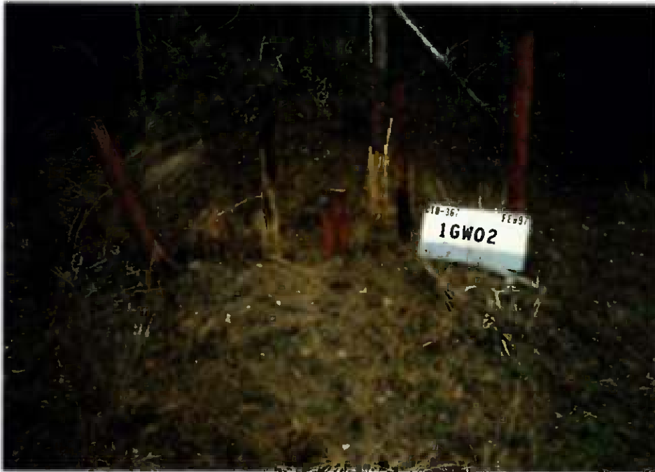
Figure 3-1 Shallow monitoring well 01-GW02 was constructed during the 1984 Confirmation Study. The well had begun to exhibit signs of neglect and deterioration.
