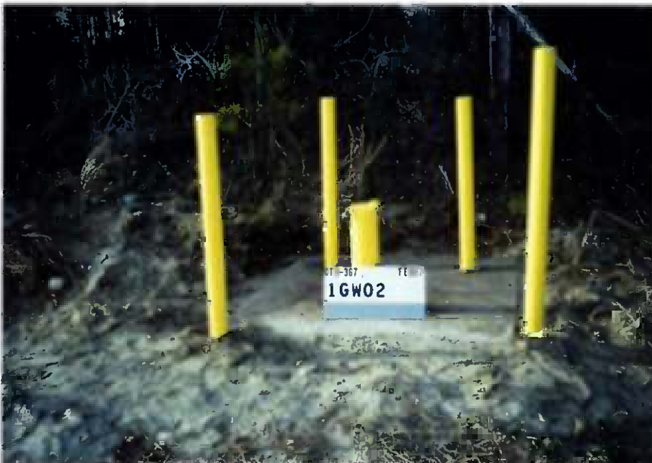
Figure 3-2 The protective bollards of monitoring well 01-GW02 were straightened and two coats of weather resistant paint were applied. A mound of soil, which had accumulated on the concrete pad, was also removed.
